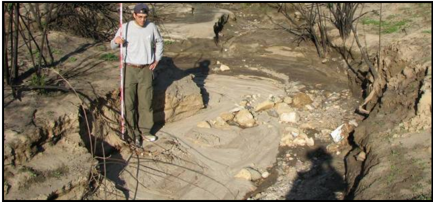
(b) Photograph looking upstream capturing interim failure of right bank
