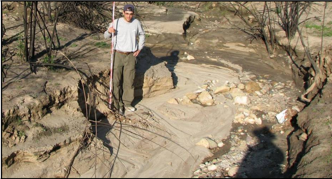
Figure 9. Bank failure at Hicks Canyon, Orange County, CA, exhibiting combinations of fluvial erosion, shallow slips, and mass failure in weakly cohesive, poorly consolidated banks.
