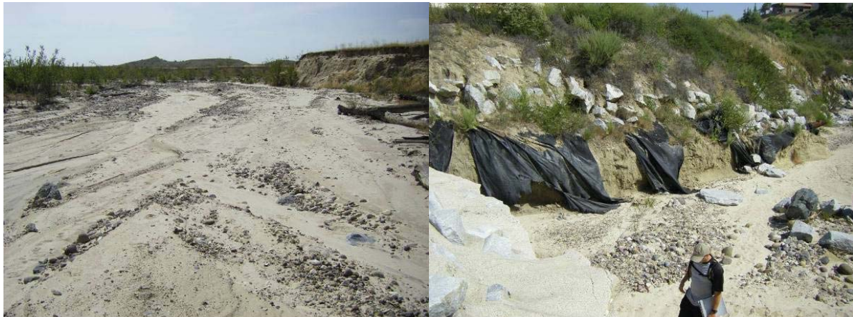
Figure 2. Alteration in channel morphology and stability, immediately upstream (left) and downstream (right) of a grade-control structure that blocks sediment passage. The two views are less than 10 m apart in the channel, with no intervening tributary.
