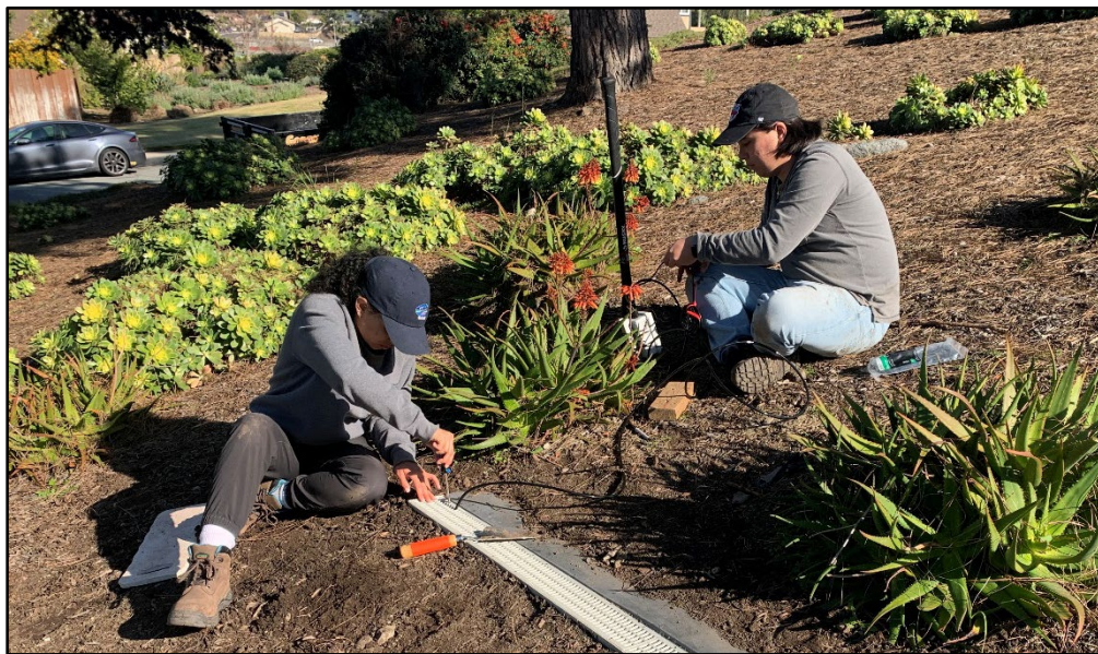
SCCWRP's Adriana Le Compte-Santiago, left, and Jerod Gray install a trench drain and above-ground sensors in a residential community where the County of San Diego replaced turf with drought-tolerant landscaping. A three-year study at this site found that replacing spray irrigation with drip irrigation and drought-tolerant plants can reduce or eliminate the volumes of irrigation and rain water running off these surfaces.
