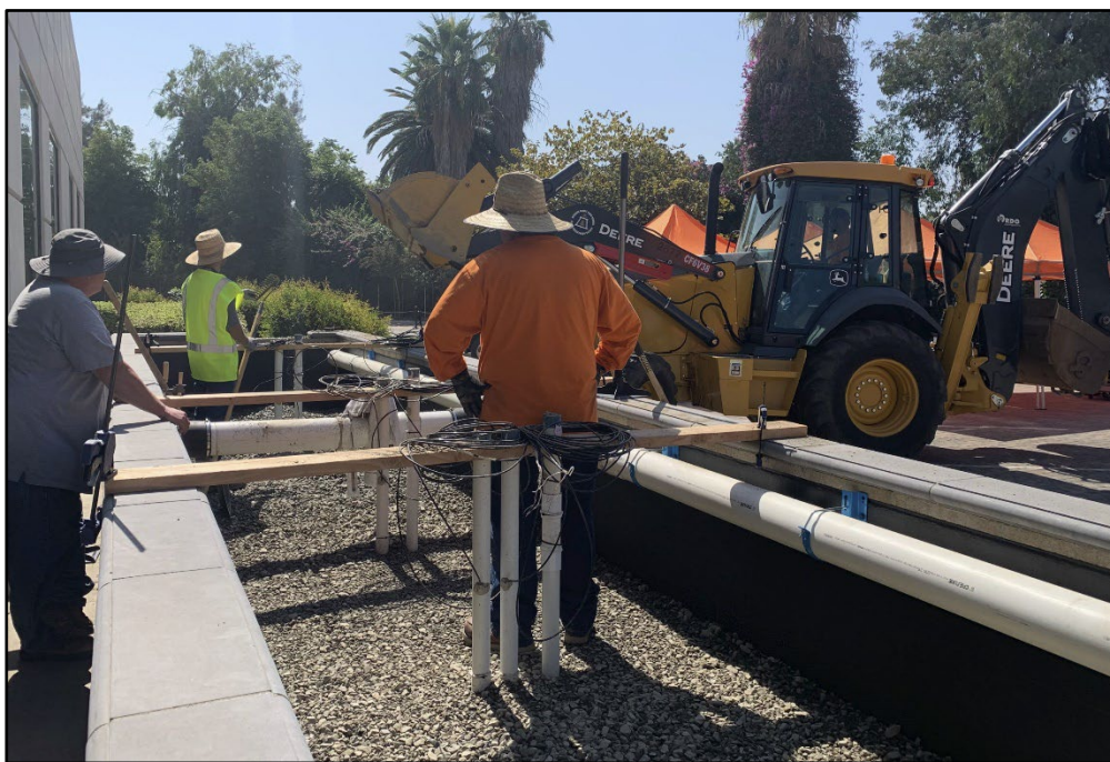
A field crew constructs a bioretention planter in Riverside County to study its mechanistic inner workings. Researchers have developed statewide guidance and a set of web tools to help California stormwater managers periodically evaluate their multi-phased plans for improving runoff water quality that have been codified into discharge permits under a philosophy known as Adaptive Watershed Management (AWM).
