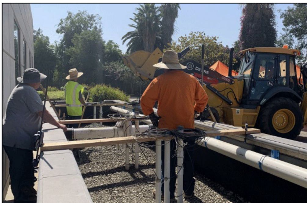
A field crew constructs a bioretention planter in Riverside County to study its mechanistic inner workings. The Southern California Stormwater Monitoring Coalition (SMC) has finalized the design of a new regional monitoring network that's being built to investigate the performance of a range of structural stormwater BMPs (best management practices), including bioretention planters.
